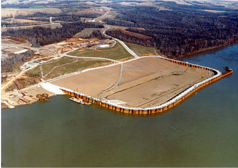
Figure I.3: Cellular sheet pile building pit for the construction of the Olmsted Locks and Dam
