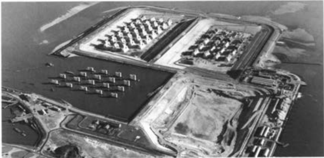
Figure I.4: Eastern Scheldt construction yards. One compartment flooded.
